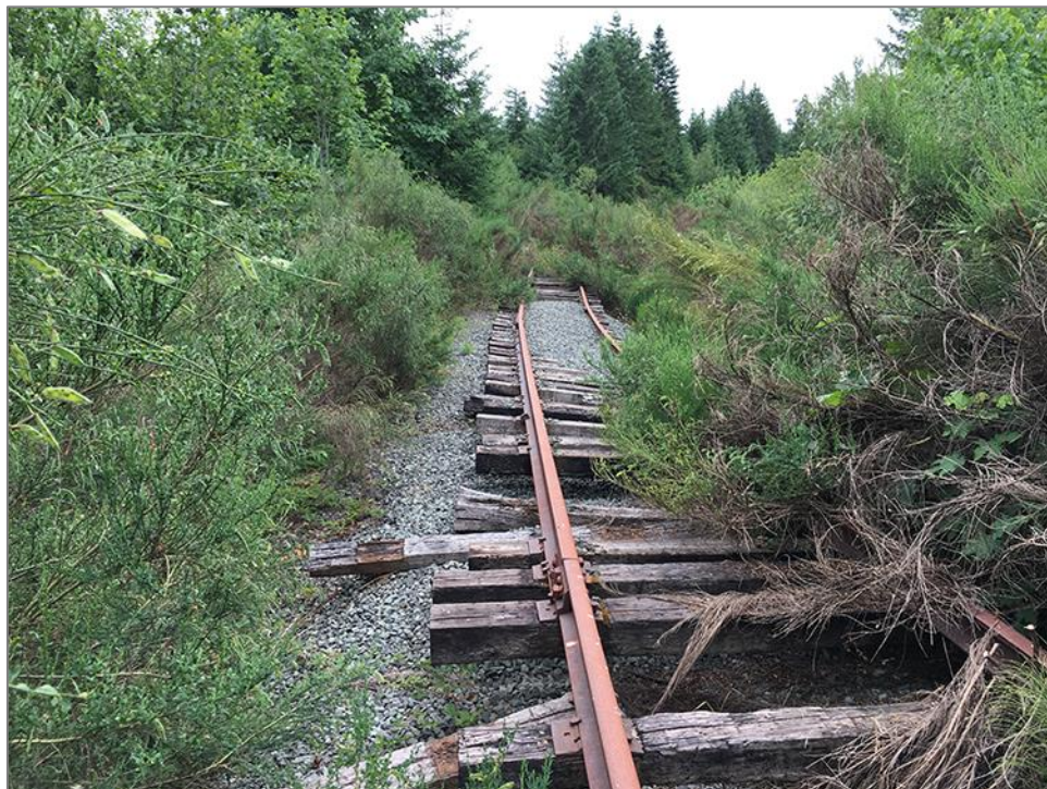
Photograph 6-17. Previously undocumented damage east of Walcott Tunnel
