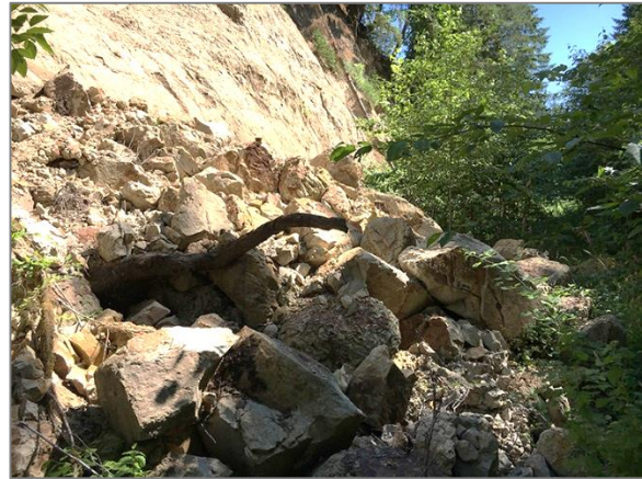
Photographs 6-18 and 6-19. Major new landslide near the OR 47 Trestle
